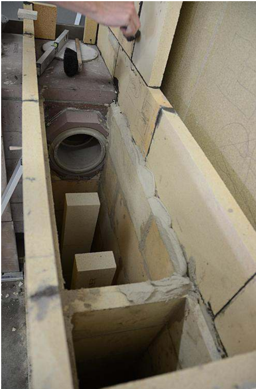
Lower bell. Firebox connection and dry-stacked columns inside the bell are visible.
